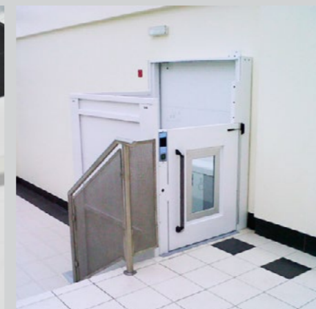
Half Height Gate at Upper Level
