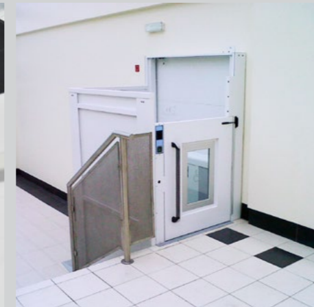
Half Height Gate at Upper Level
